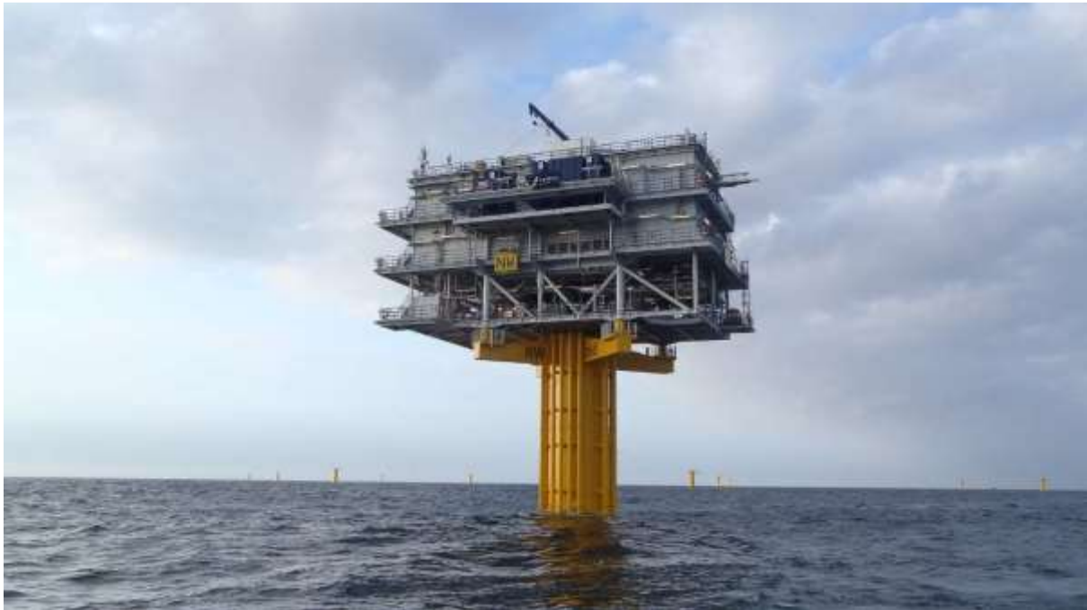
Figure 2.8. Offshore substation on Princess Amalia Offshore Wind Farm [Source: https://isc.dk/en/northwind-vindmoellepark/ ]
